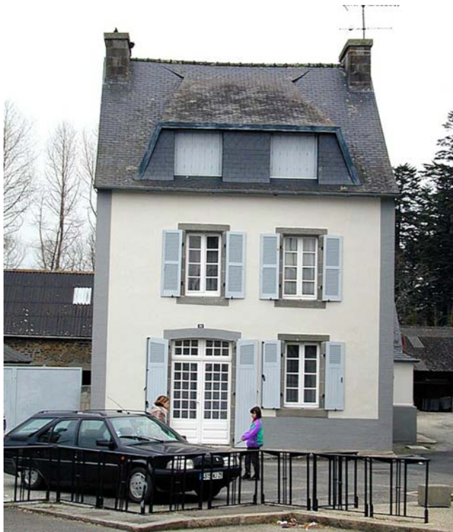
Figure 20. This house in Bretagne has mosses invading the roof. Photo by Michael Lüth.
